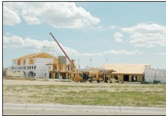
Outlook photo by Larry Tanglen High Tech Construction workers place roof trusses in place at the main apartment building of The Crossing, a senior living complex being built by St. John's Lutheran Ministries, off of East Maryland in Laurel. It is slated for completion and occupancy later this year.
