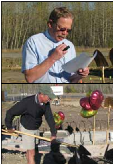
Above, Pr. Kim Wilker lead prayer at the Foundation Blessing at The Willows. Below, St. John's Board Member and Red Lodge resident Jiom Ochiltree shovels concrete into a footing.
