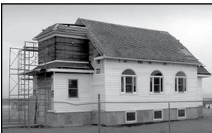
Photo shows new windows and siding on the south side of the church.
