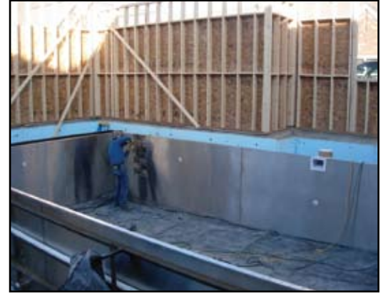
The foundation has been poured and the swimming pool begins to take shape.
